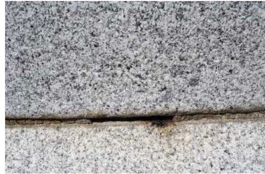
Figure 33 The joints should be repointed with a lime mortar to match the existing.
