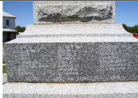
Figure 35 The joints should be repointed with a lime mortar to match the existing.
