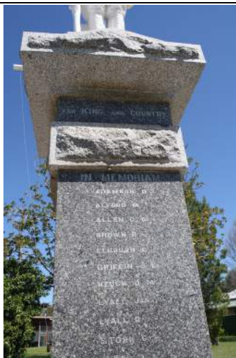
Figure 36 Washed stone with a soft brush and water and a low ph soap if required.
