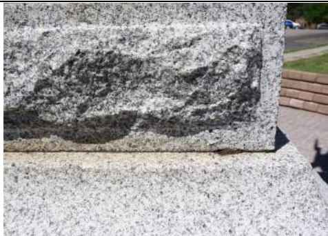
Figure 34 The joints should be repointed with a lime mortar to match the existing.
