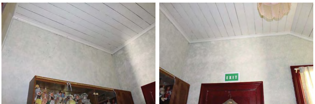
Figure 43: Views of the timber board ceilings with the southern portion of the Store Rooms.
