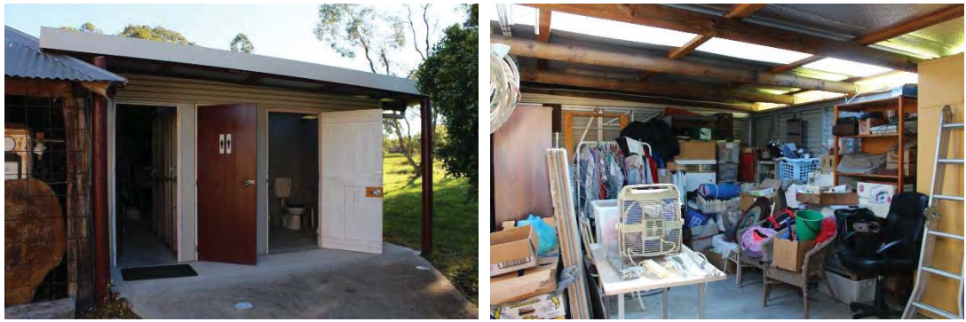
Figure 48: View of the northern addition constructed in 2013, attached to the northern elevation of the central portion of the Outbuilding (left) and view inside the storage room which lays directly behind the toilets (right).
