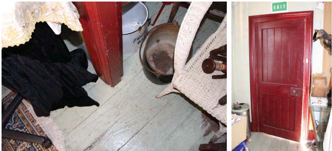
Figure 40: Painted timber floorboards in the Store Room (left) and view of the interior of the ledged door, located on the northern wall of the Store Room (left)
