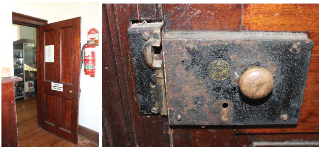
Figure 34: Internal four panel timber door with original hardware, located on the northern wall of the Police Office.
