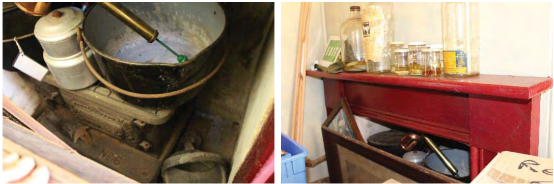
Figure 39: View of the cast-iron stove within the fire-place of the Store Room (left) and view of the top portion of the timber fireplace surround in the Store Room (right)
