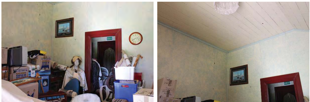
Figure 37: View of the inserted partition wall which divides the Store Room space into two rooms (left) and view of the ceiling within the northern portion of the Store Room (right)
