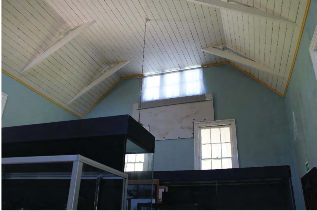
Figure 28: View of the trapezium tongue & groove timber boarded ceiling with exposed purlins and decorative timber brackets in the Court Room.
