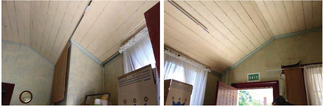
Figure 38: View of the chimney breast and western wall of the Store Room (left) and view of the northern wall of the Store Room (right). Some of the plaster from the north wall is failing, located to the left of the window.
