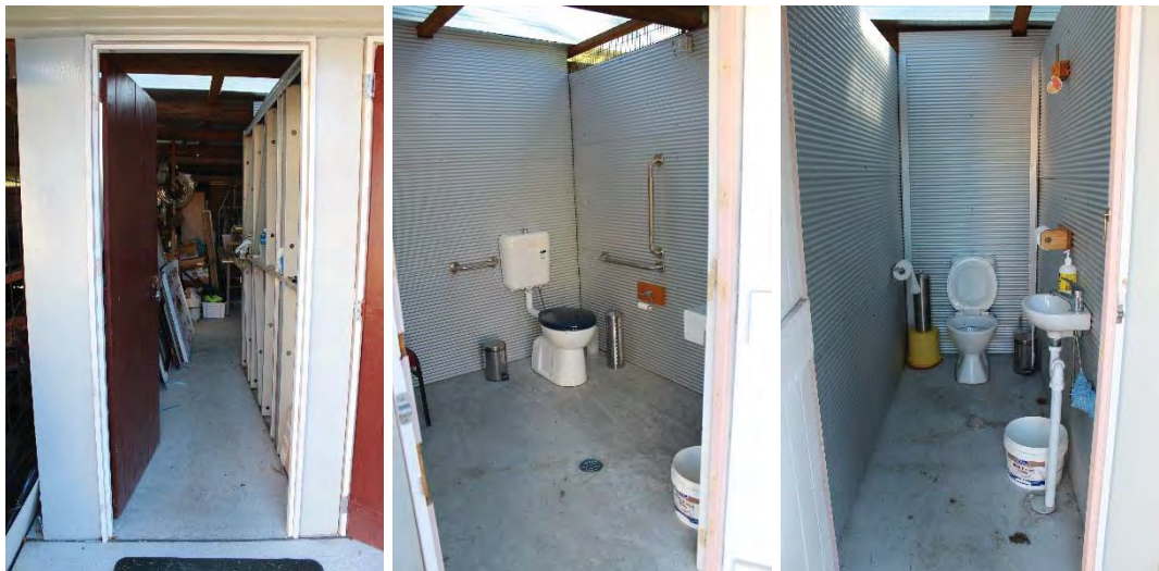
Figure 49: View of entry into the storage room which lies directly behind the bathrooms within the northern addition (left), interior view of the disabled toilet (middle) and interior view of the unisex toilet (right).
