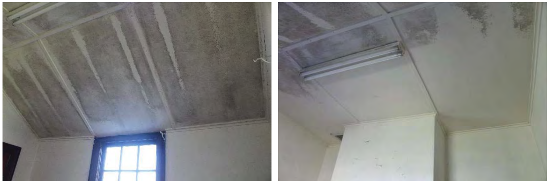
Figure 33: Plasterboard and batten ceiling of the Police Office, showing signs of water ingress with extensive mould.
