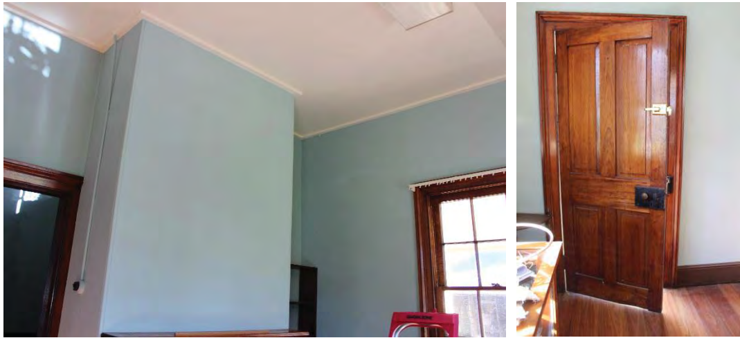
Figure 36: View of the plasterboard ceiling in the Magistrate's Room (left) and interior view of the external door in the Magistrate's Room, which leads to the verandah (right)
