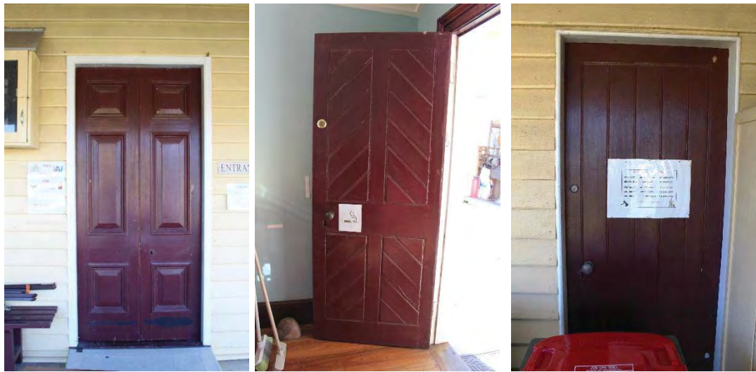
Figure 26: Three different types of external doors at the Courthouse: six panel double-leaf (left); four panel (middle) and ledged (right)
