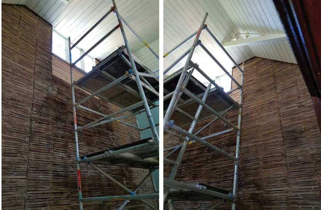
Figure 130: Western wall of Court Room during the maintenance works. All original plaster was removed from the laths with new laths being installed under and to the right of the western gable windows (Source: Dianne Ellis, Clarence Town and District Historical Museum Committee)
