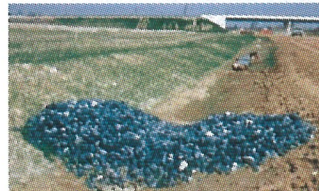
CHECK DAM EXAMPLES MORE INFORMATION ON CHECK DAMS IS AVAILABLE IN THE TOWN CREEK PLAN OF MANAGEMENT - 'APPENDIX B'
